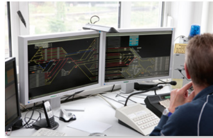
Central operating workstation
